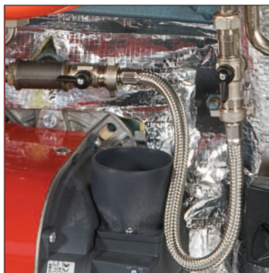
Filling Loop fitted in boiler.
