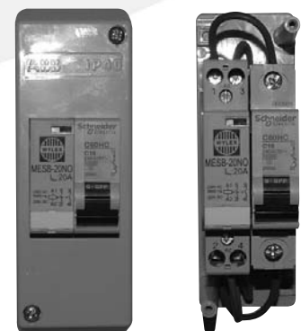
Figure 9-3: HW booster kit with cover removed to show relay
