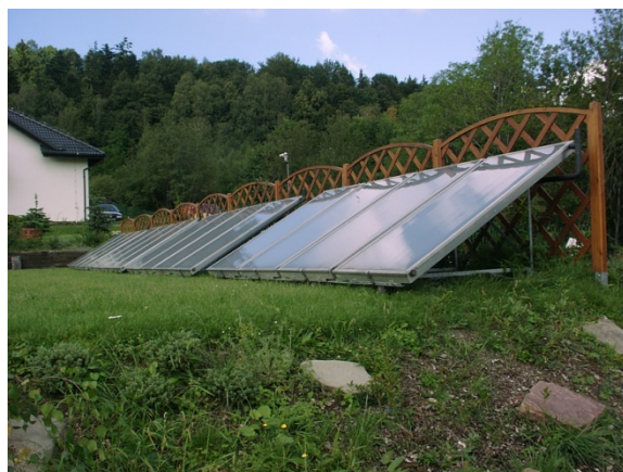
Figure 4 Ground mounted on 'A' frame.
