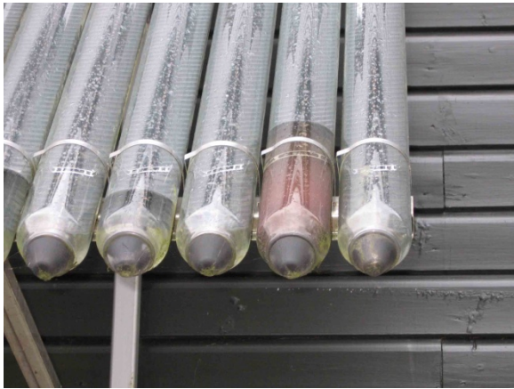
Figure 18 Tube seal failure
