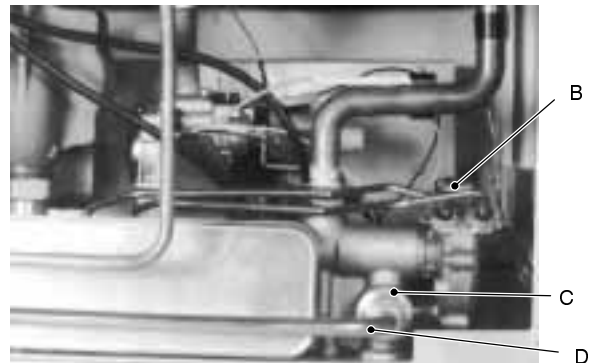
fig. 69 (rear view of the boiler)
