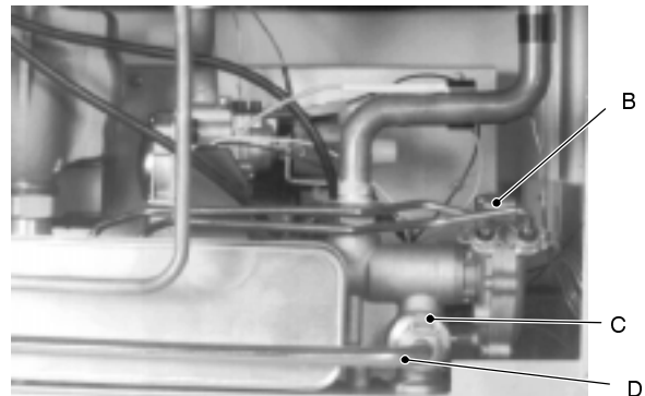
fig. 75 (rear view of the boiler)
