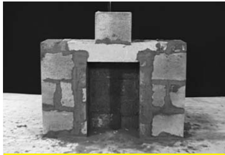
8 The first chimney block is now set on a bed of mortar on top of the lintel. The insulation and Ceramic liner are inserted in the standard way.
