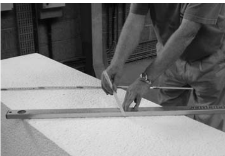
7 Now draw the angle of the roof slope across the prefabricated stack.
