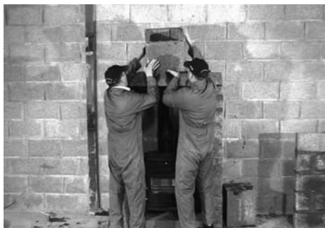
5 Place the chimney block on a support block on a bed of mortar.
