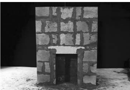
13 Continue to build the chimney breast with chimney blocks and hollow blocks, inserting the flue liners and insulation until the top of the chimney breast is reached.
