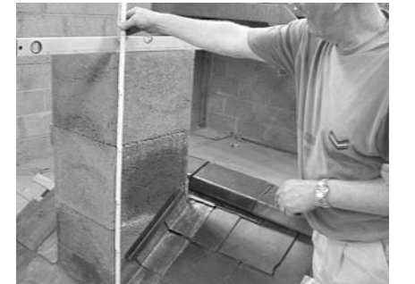
3 Carefully measure the height of the leading edge of the chimney stack.
