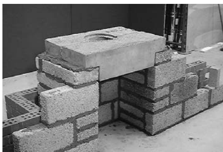
4 Place the lintel marked FRONT (larger) beside the back lintel, on a bed of mortar.
