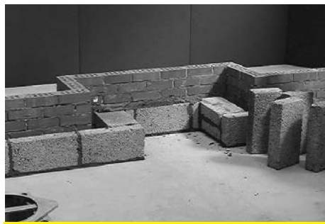
1 The fire chamber should be built in the traditional manner. The inner and outer blocks or bricks are built on a suitable foundation. The outer brick or block work should be at least 6.5 brick by 2 brick wide (1460x450mm).
