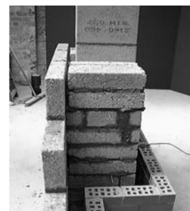
6 Place on the first chimney block so that it is flush with the inside of the cavity. The insulation and ceramic liners should be added in the standard way. Place standard concrete blocks either side of the chimney block. Cavity wall ties should be used to tie the chimney to the outside skin.
