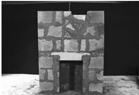
10 To complete the kit place the 2 triangular cut blocks and the last half hollow block. This gives a horizontal offset of 200mm.
