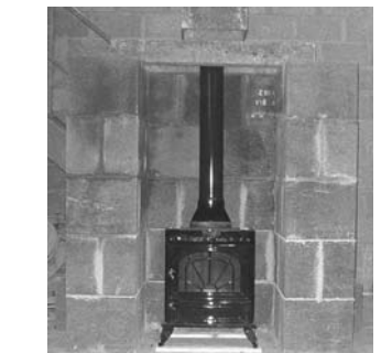
6 The chimney is then built in the standard manner as a single block.
