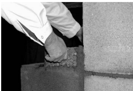
14 Place 6 concrete blocks over the blocks at the top of the chimney breast.
