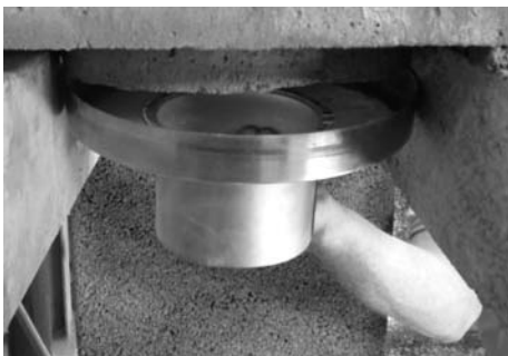
4 Secure the metal adaptor to the under side of the support block.
