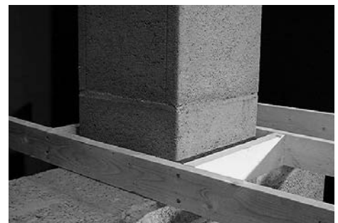
15 Where the chimney passes through floor or ceiling joists, these need to be trimmed out leaving a gap of 40mm for timber and 30mm for concrete. This gap is then filled with non-combustible material..
