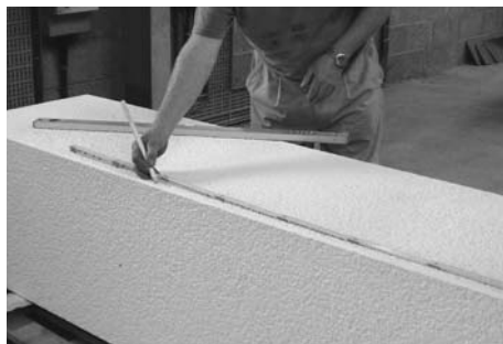
5 Mark out the bigger height on one edge of the prefabricated stack, measuring from the top of the prefabricated stack.
