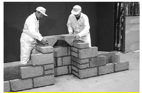
3 Place the lintel marked BACK (smaller) in position, on a bed of mortar. Apply the high temperature sealant on the inner side of the lintel.
