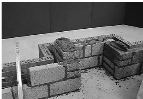
2 The fire opening should be 600mm(24") wide by 550mm(22") to the back of the cavity. The blockwork piers should be built on their flat side to a height of 750mm from finish floor.
