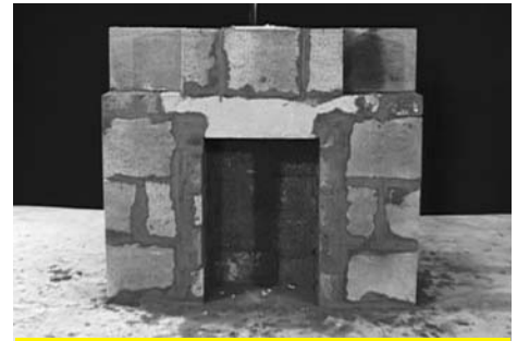
9 The chimney breast is formed either side of the chimney block by using the hollow blocks.
