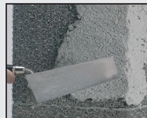
We recommend plastering the block to seal the chimney.
