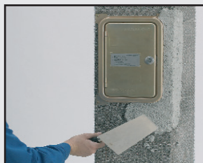
Plaster around the cleaning door.
