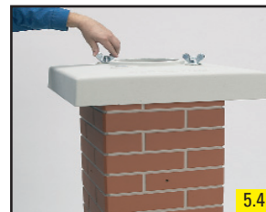
5.4 Screw on the coping, free holes to be closed with plastic caps.
